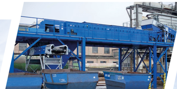
STEINERT SteelMaster in an end-of-life vehicle recycling plant in the UK
